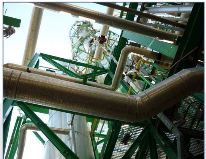
Fig. 1 - Oil and gas treatment plant
