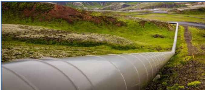
Fig. 4 - Crude export pipeline
