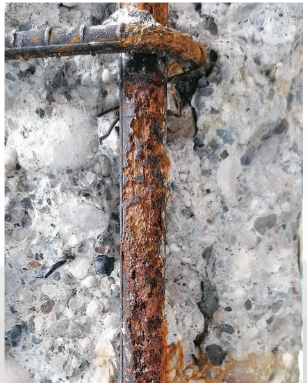
Fig. 1 - Example of corrosion attack on a rebar
